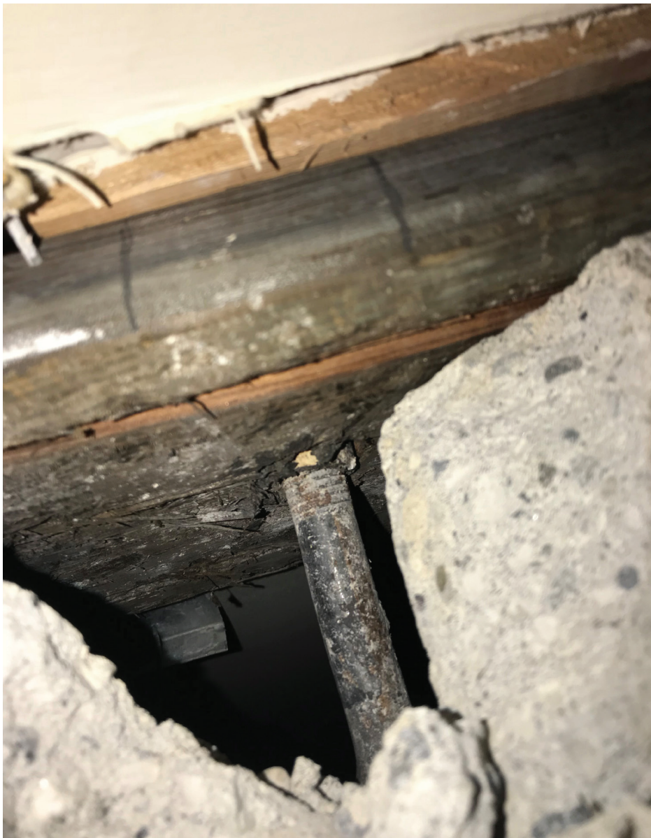
Figure 2. Top of CMU Wall Damage
