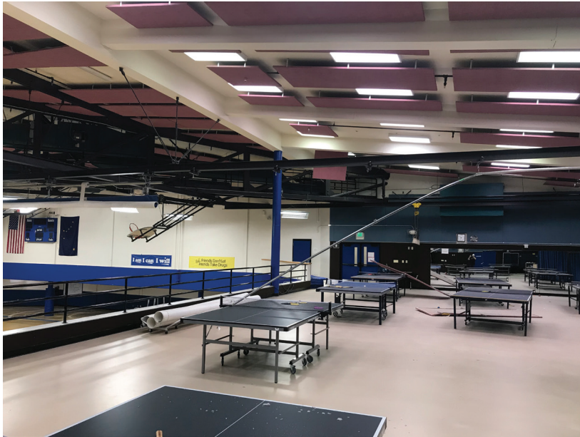
Figure 3. Damaged Curtain Support Beam
