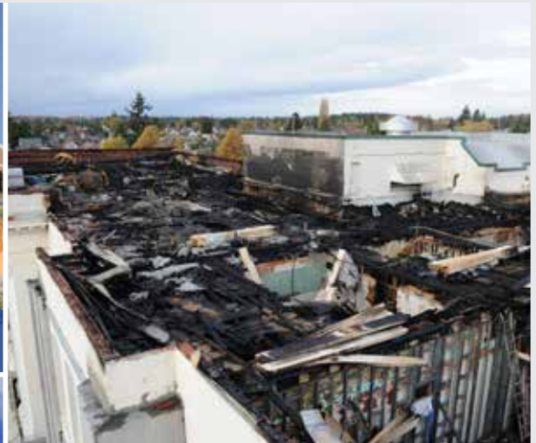
Whatcom Middle School Post-Fire, Bellingham, WA
